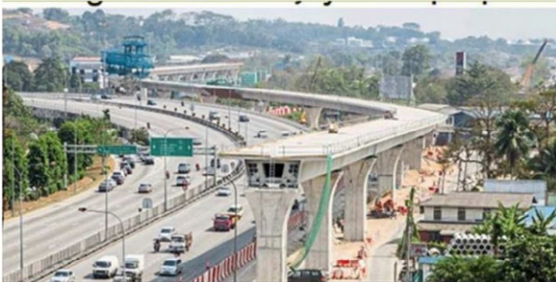
MRT Corp's Sungai Buloh-Kajang Line. MRT Corp has proposed a new alignment option for the Sungai Buloh-Serdang-Putrajaya Line which needs to get approval first.
